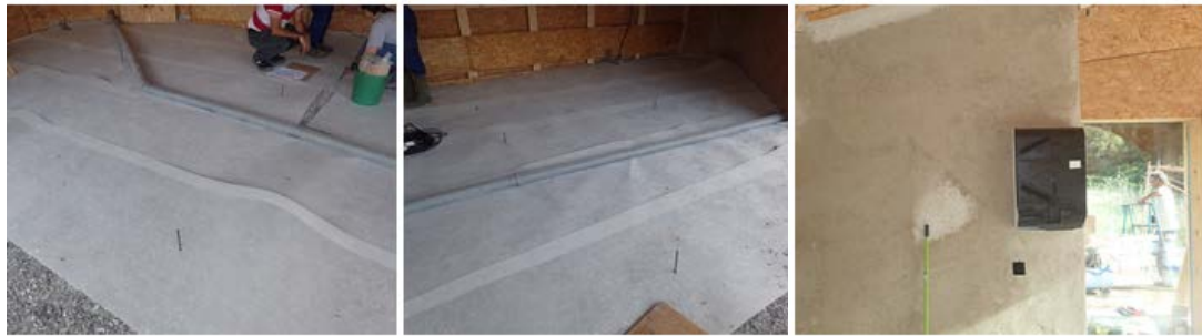
Figure 6. Placement of air ducts for the heat exchanger (left and middle). The heat exchanger installed (right).
