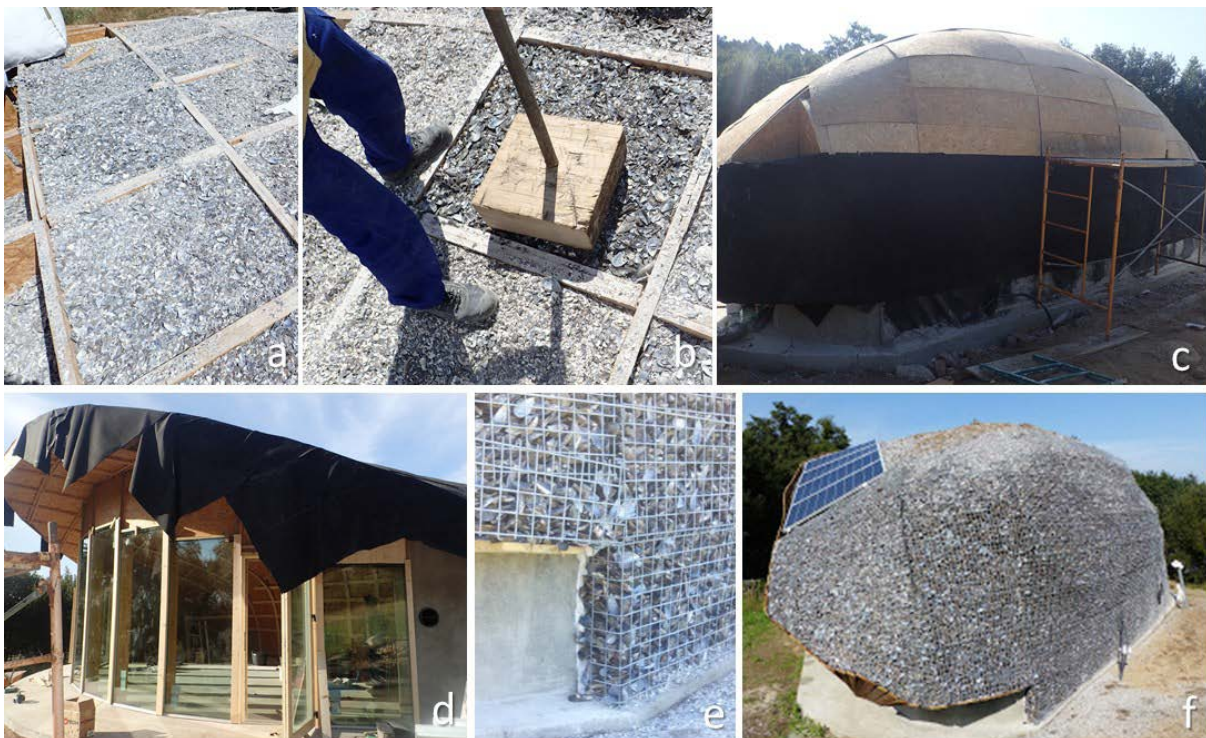
Figure 13. Constructive process of the roof: a) mussel shells inside roof structure compaction of mussel shells, b).
