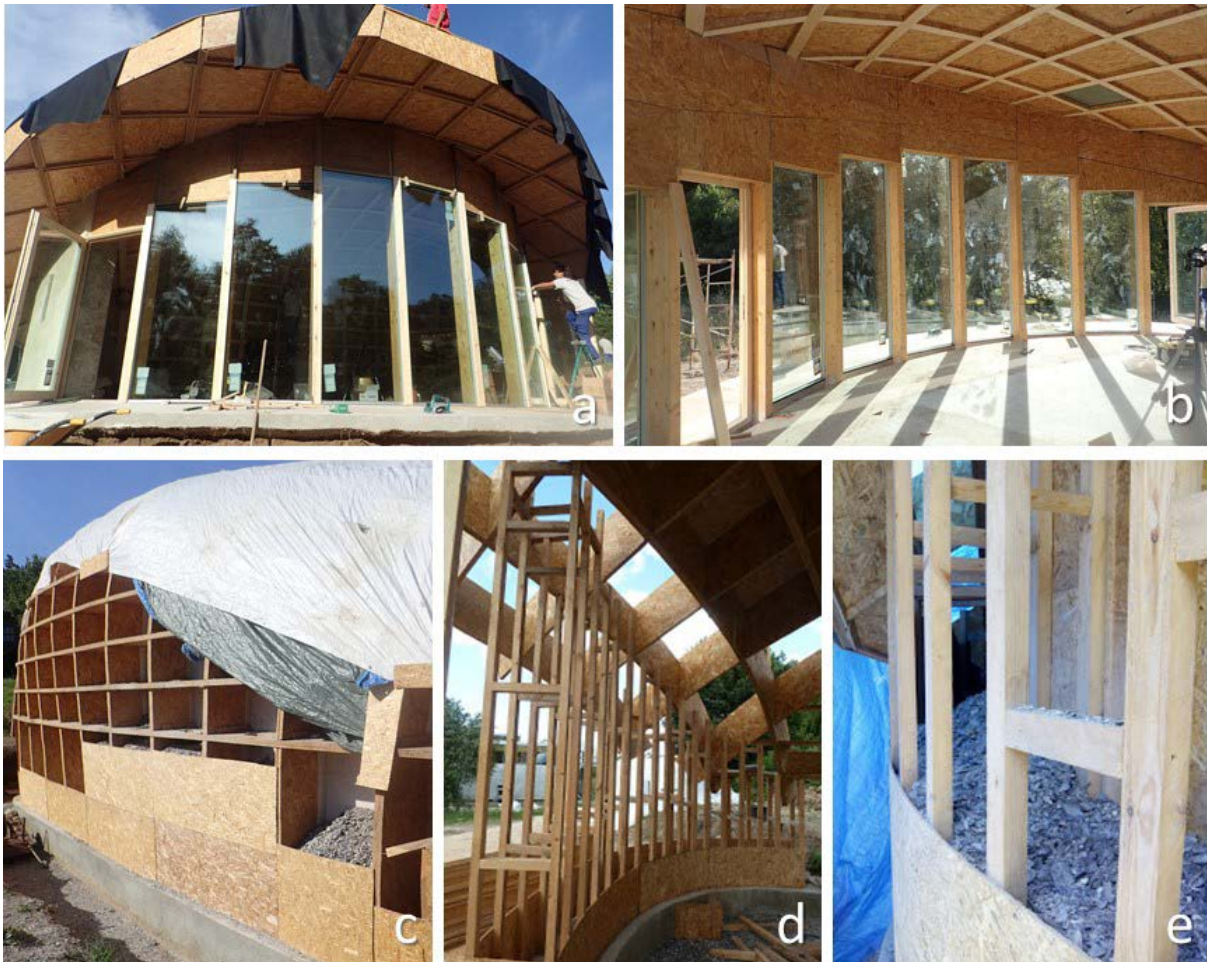
Figure 15. Constructive process of façades and walls: a) glazing façade, b) interior view of glazing of windows and doors, c) vertical roof with loose-fill made of compacted mussel shell gravel, d) NW timber wall structure, e) application of loose-fill insulation in wall.
