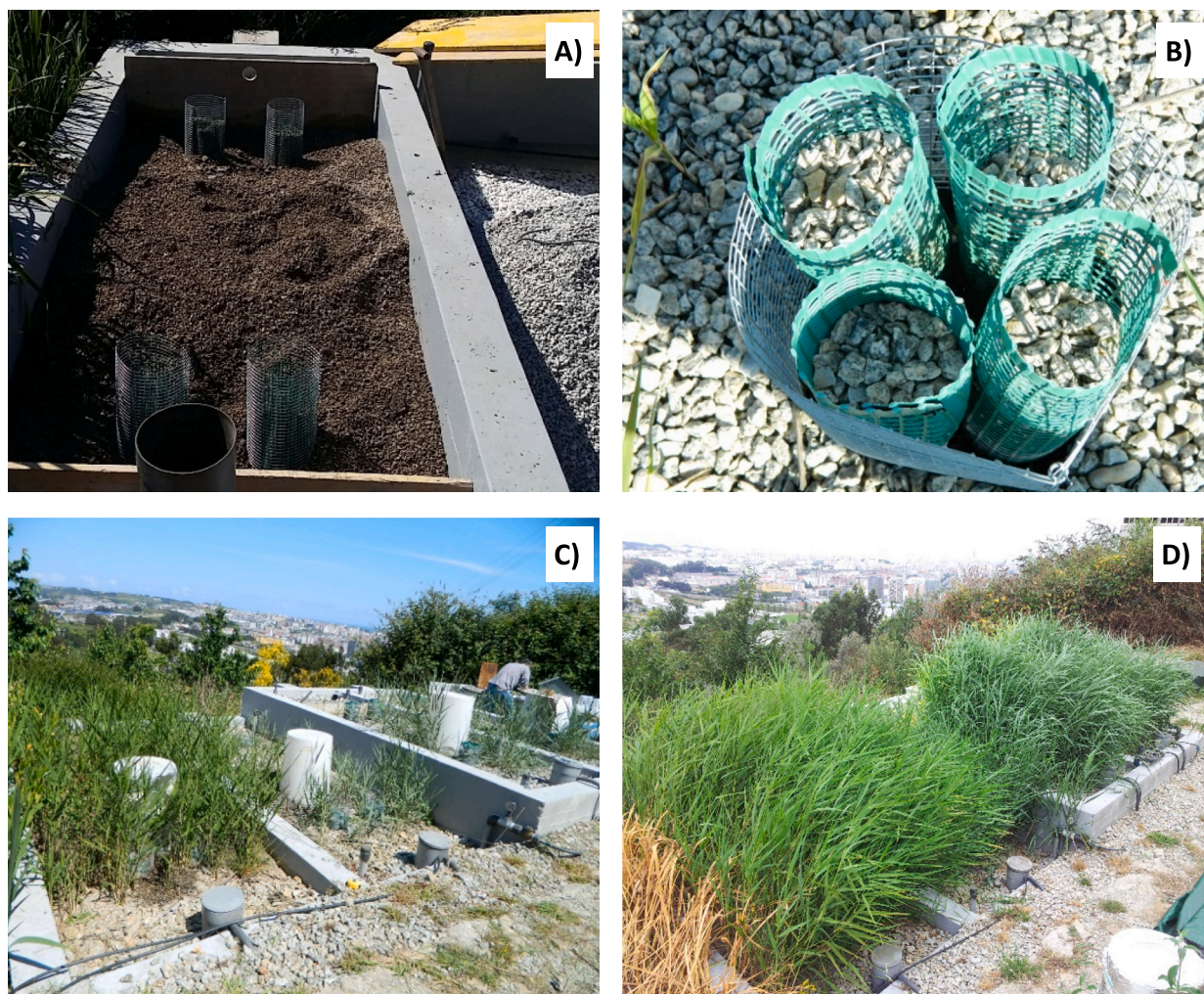
Fig. 2. Construction details (A, B), plastic chambers during gas emission campaigns (C) and view of the planted units (D).
