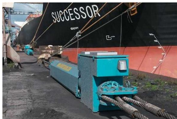
Fig. 12 – Hydraulic mooring system. Source: KRVE (2016)
