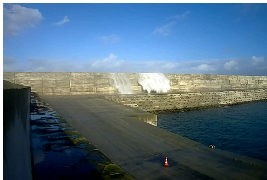
Figure 2. Overtopping example. Outer port of Punta Langosteira, A Coruña, Spain.
