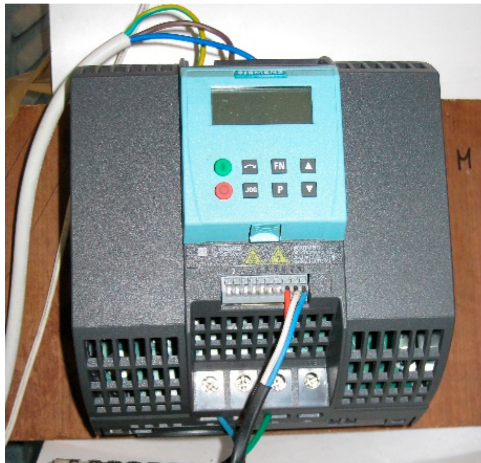
Figure 11. Ventilator and speed control system (Siemens Sinamics G110).
