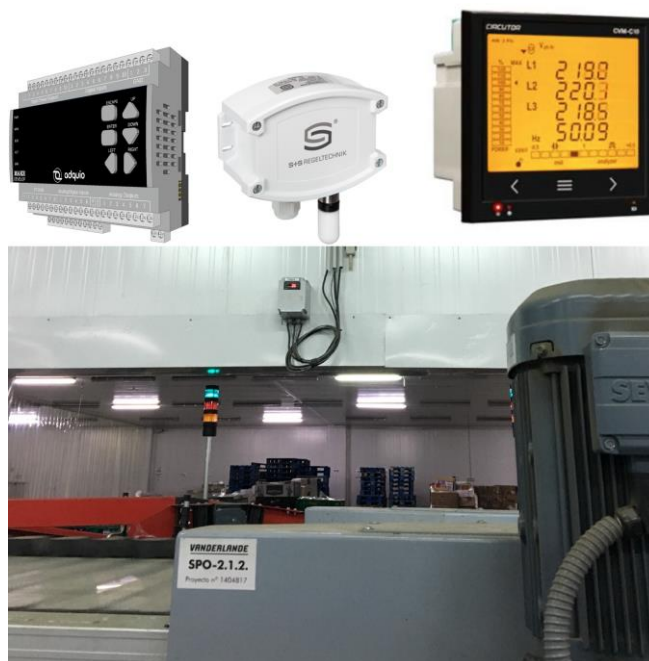
Fig. 2. Hardware used for monitoring the facility. Top Left: Adquio Pro programmable controller. Center: Regeltechnik ATF temperature controller. Right: Circutor CVM-C10 network analyzer. Bottom: Sensors in the actual facility. See the main text for a detailed explanation.
