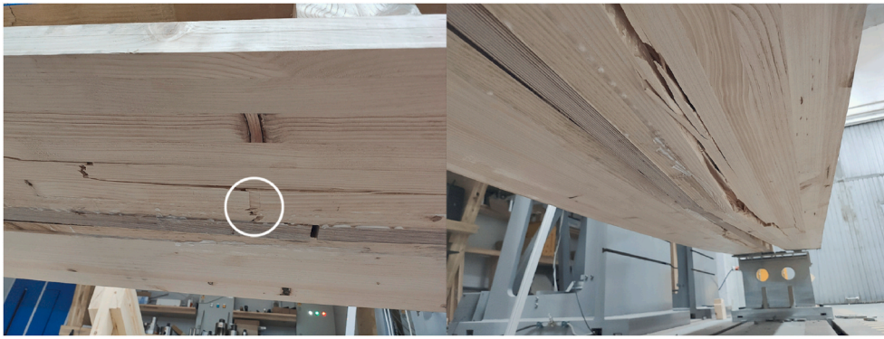
Fig. 7. Photographs of the underside of the glulam flange at the end of tests 250.2-B and 300.1-C. On the left, a break initiated in a finger joint (near one of the plywood rib discontinuities) can be seen.
