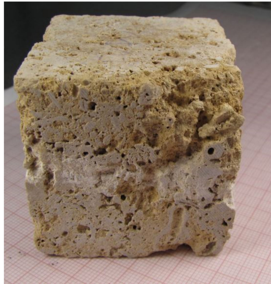
Figure 2. Limestone (travertine) after cycles of salt crystallization with sodium sulphate solutions (note the accumulation of salt efflorescences and the existence of irregular erosion patterns in relation to the shape of the specimen and the rock texture).
