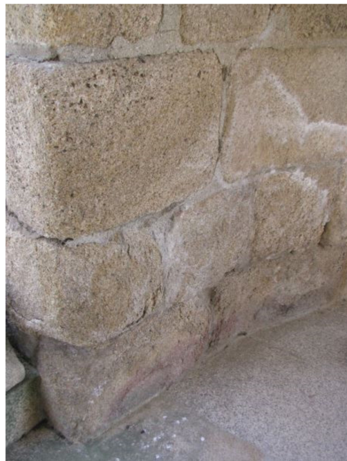
Figure 1. Salt efflorescences (whitish powder) and erosive effects (leading to rounding) on granitic stones of a window from a historical structure in the town of Chaves (Portugal).
