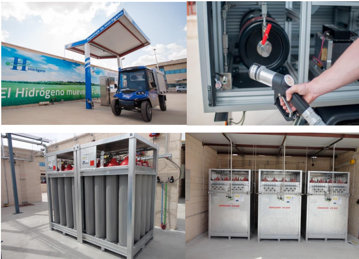
Figure 6. Real installation of both H2 Storage and the Application of it on Vehicles in Ciudad Real- Spain.
