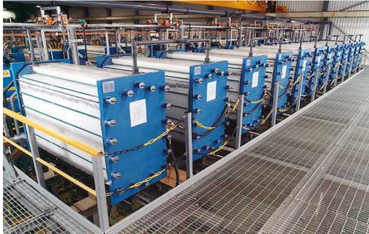
Figure 32. Redox Flow Batteries. Lancaster, NY.
