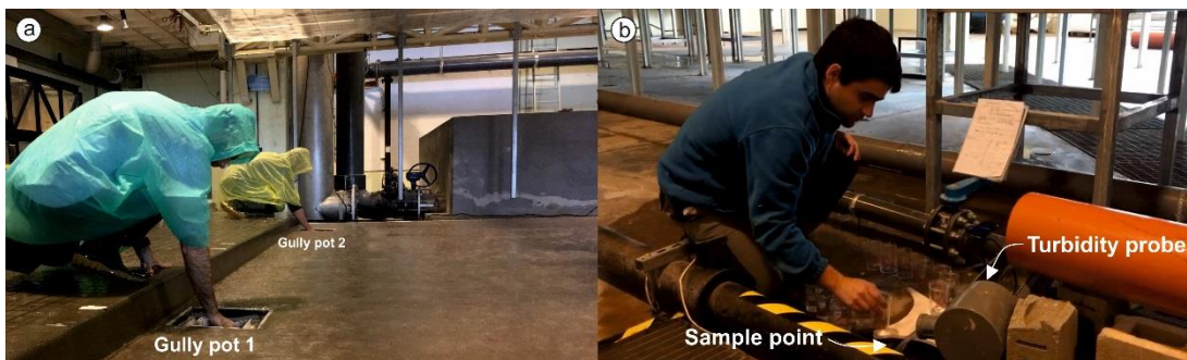
Figure 5.13. PSD and TSS samples measuring points at the entrance of gully pots (a) and at the pipe system outlet (b).
