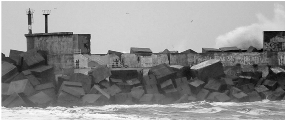
Figure 18. Displacement of the upper part of the crown wall in the breakwater of A Garda, Spain (2017).
