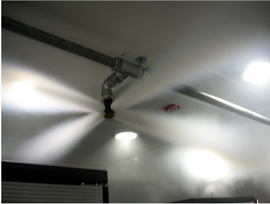
Figure 1.11: Discharge of HFC-227ea agent in a protected room.
