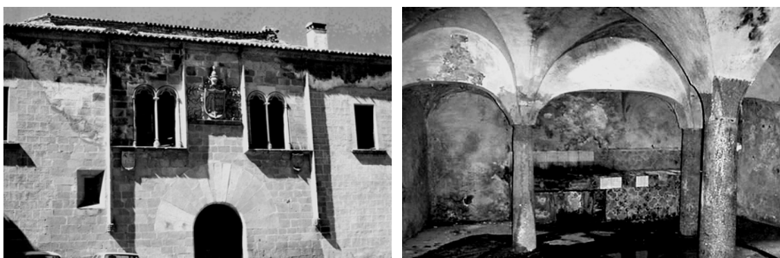
Figs. 4 and 5. The building was strongly degraded: main facade (left) and old kitchen (right).
