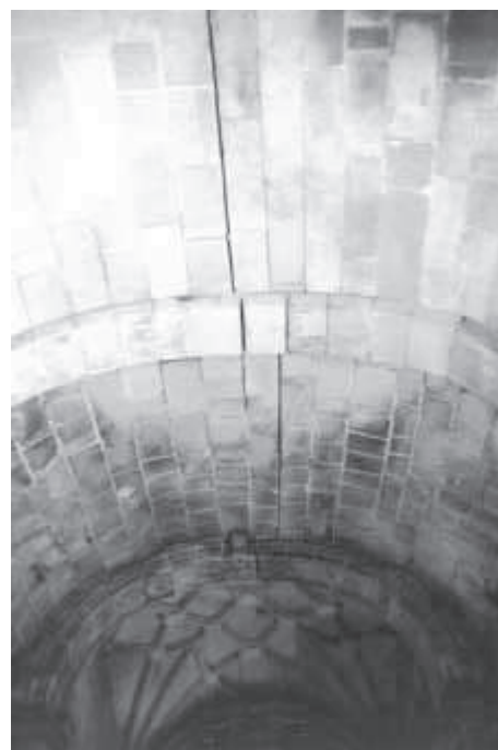
Figure 6 : Grietas in the vault
