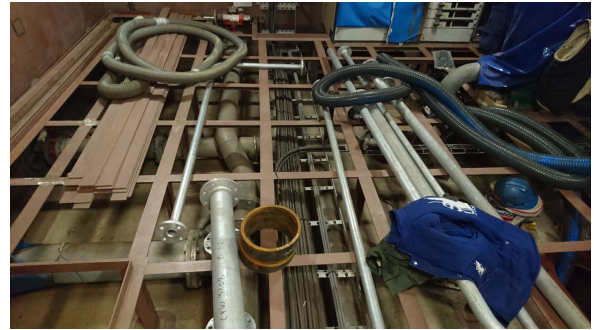
FIGURE 5. Pipes under metal floor.
