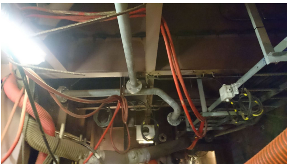
FIGURE 4. Mounted pipes on the ship ceiling.
