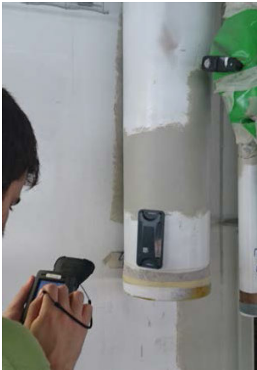
FIGURE 10. Testing of a passive RFID tag attached to one of the main pipes of the ship block.
