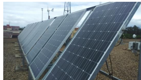
Figure 7: Aspect of the set of PV modules.
