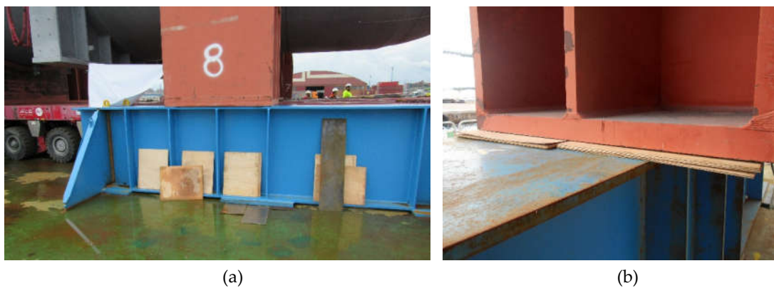
Figure 10. (a) Cradle in the position just over the three stiffenings. The two stiffenings of the beam-ends aligned with the bearing plates. (b) Plywood as dunnage placed in the void space between the cradle and the grillage beam.
